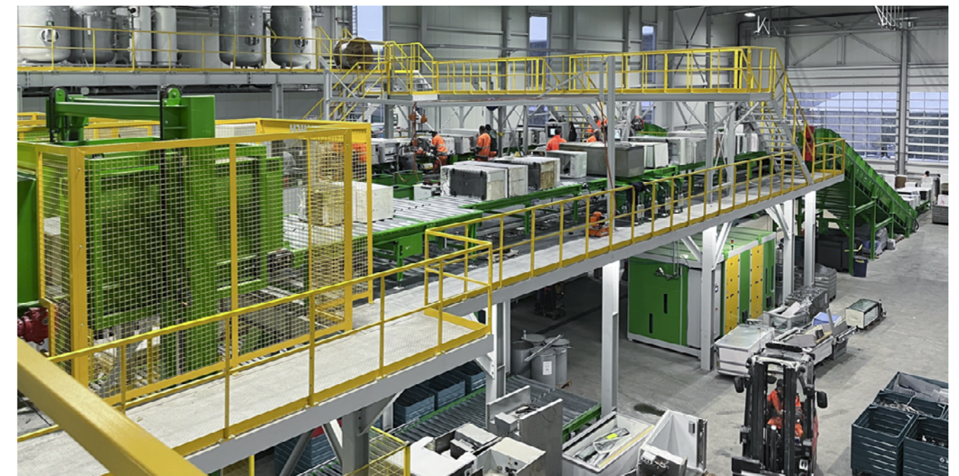
Erdwich refrigerator recycling plant of Immark AG. Middle: upper plant deck with extraction stations, left: appliance infeed in the second processing stage, with the N2 production plant in the background.
